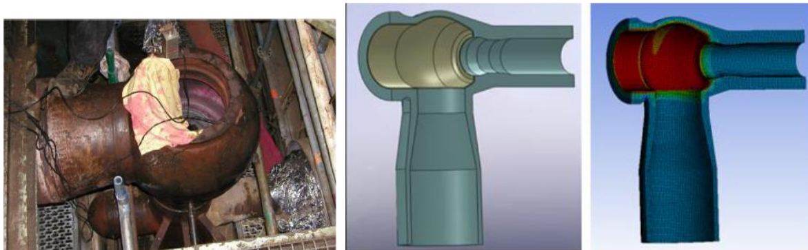
Figure 1.17 Left: Photo of valve during inspection. Right: Stress distribution in valve.
