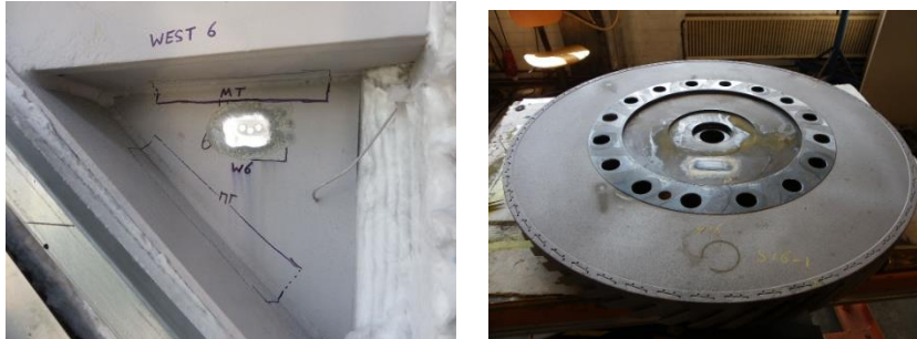
Figure 1.51 Areas for hardness measurements. Left: boiler components that have been temporarily overheated. Right: gas turbine disc. As surface preparation is needed for HT and for replication, these tests are normally done at the same position.
