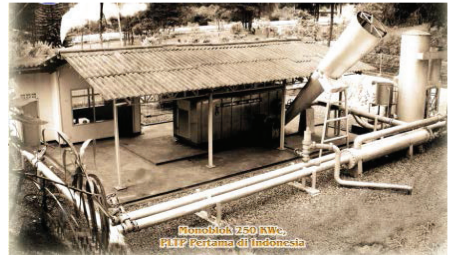
Figure 10 Monoblok 0.25 MW Power Plant (1978) source: courtesy of PGE
