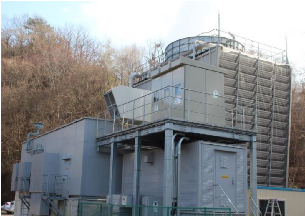
Figure 8: Waita geothermal plant, Japan
