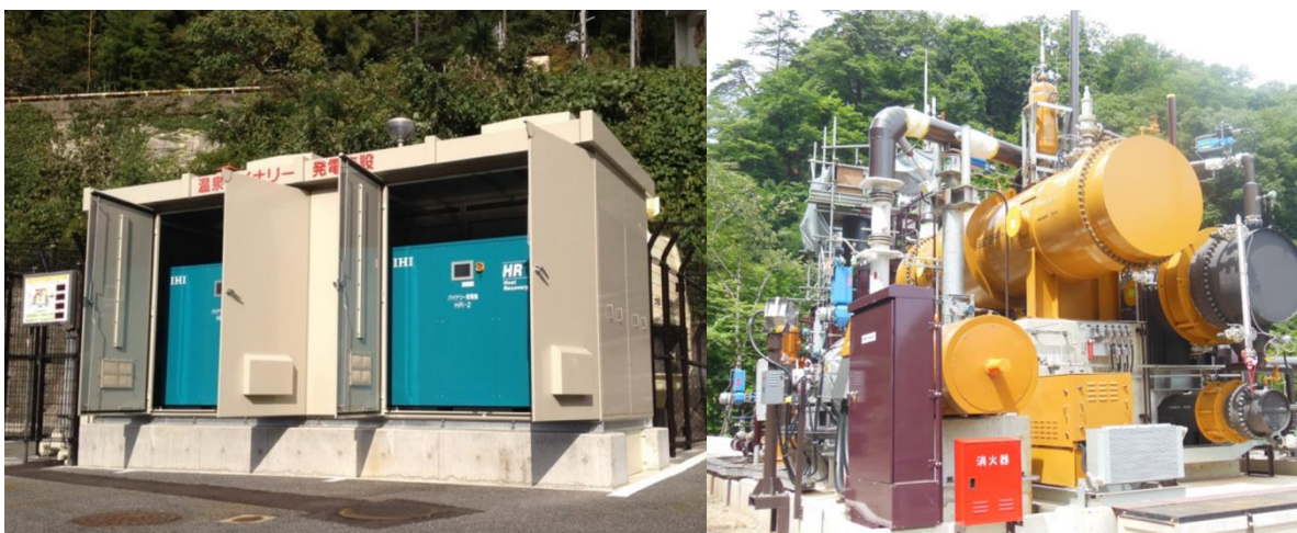
Figure 4: left: Onsen Binary Geothermal Systems (2 x 20 kW), Credit: The Town of Shinonsen; right: 400-kW Onsen Binary Geothermal Power Plant at Tsuchiyu, Fukushima Prefecture, Credit: Genki Up Tsuchiyu Company
